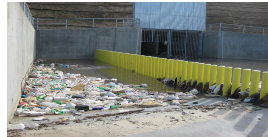
Photos depict debris/silt deposits in Smuggler's Gulch and Goat Canyon after major storm event on Dec 6 th , 2009
