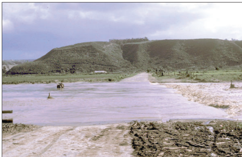
Figure 2. In 1980, the Tijuana River flood washed out 19th Street in Imperial Beach, California; as a result of recurrent flooding this was never repaired.
